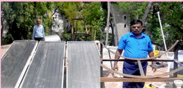
M/s Sharon Solar Solutions, Thiruparangundram, Madurai.
